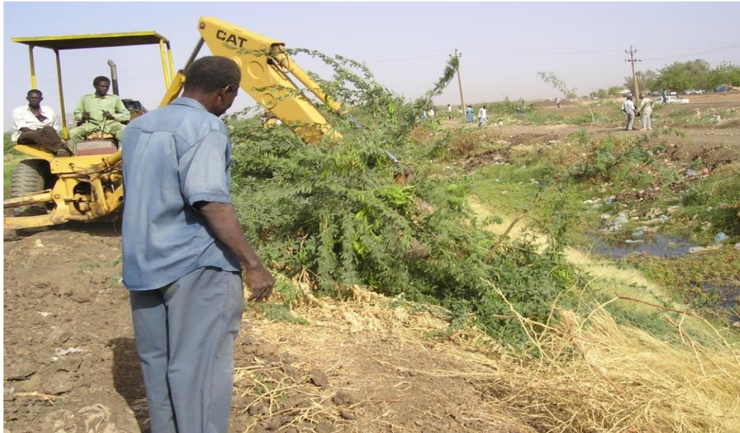
Figure 5.8 Mechanical and heavy equipment method can be used as in New Halfa scheme
